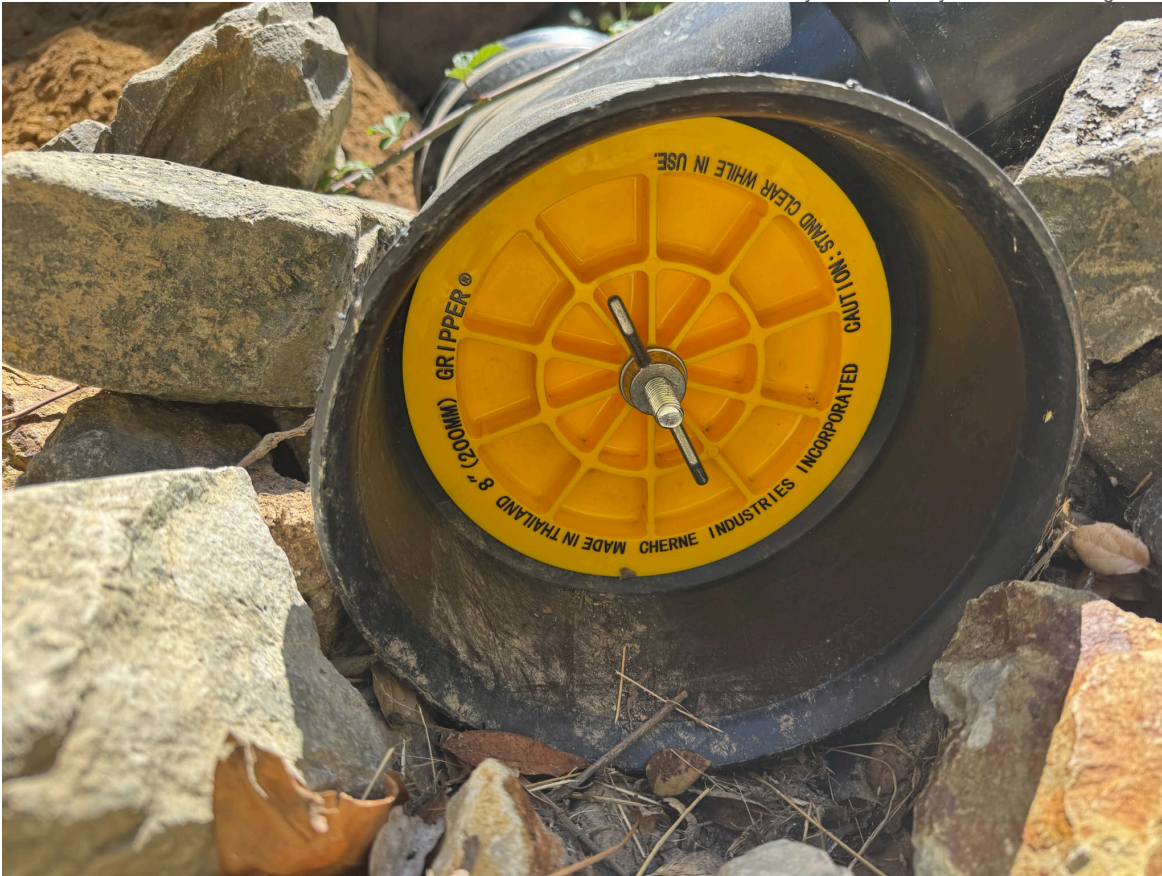
Photo 1. Installed pipe termination detail with removable gripper-style plug/cap visible inside drainage pipe.
