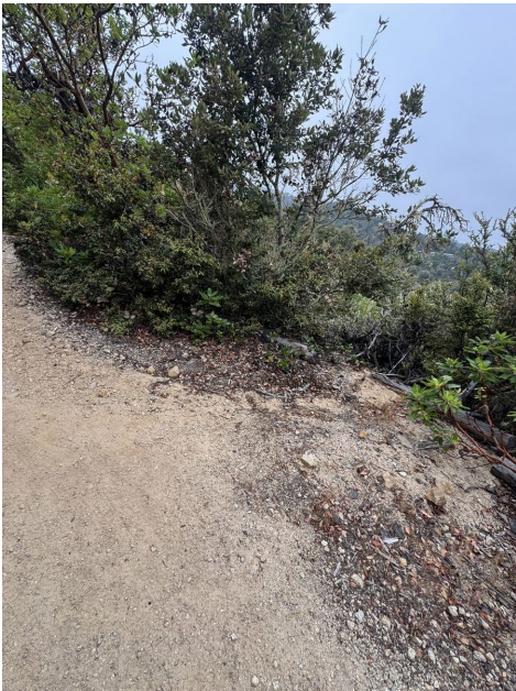
Photo 5: Failed water bar
