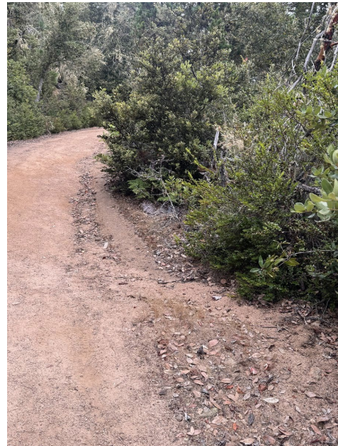
Photo 6: Failed water bar
